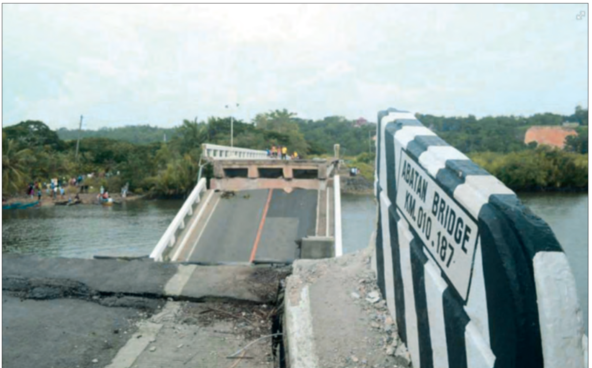
Figure 6d: The destroyed Abatan Bridge that connects Maribojoc to Tagbilaran City, the capital of Bohol
